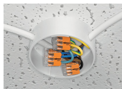
Lighting distribution in a ceiling canopy
